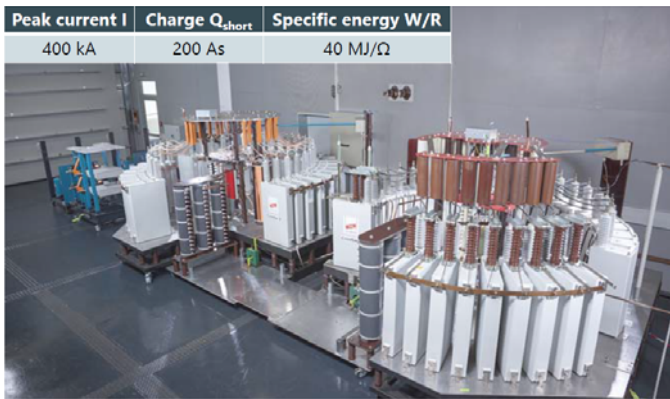
Figure 4 : Extreme high lightning currents generator.
