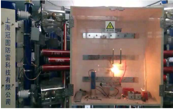
Figure 16 : picture shows that the SPDs is under fire
